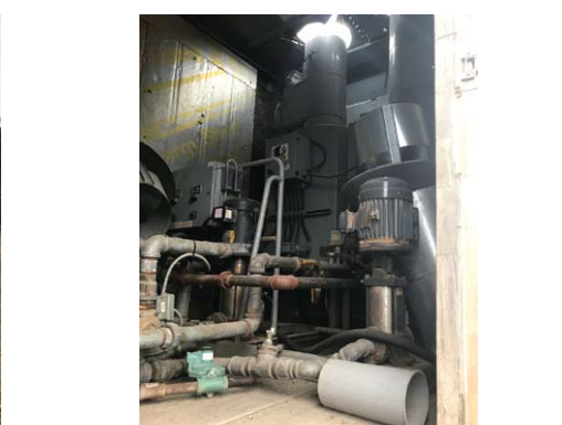
2,000,000 BTU Heater in Trailer
